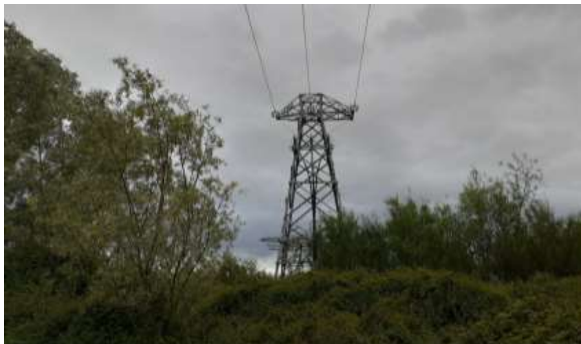
Figure 4-61: Overhead ESB utilities
