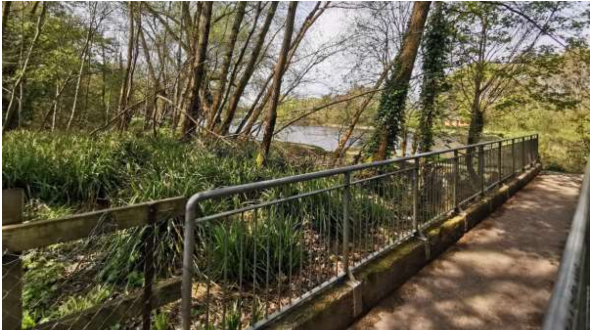
Figure 4-49: Existing concrete bridge at mouth of Plassey mill race with Plassey Beach in the background
