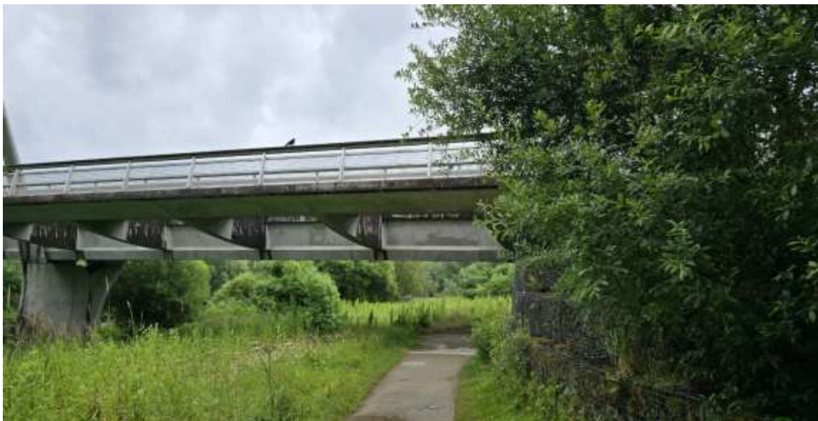
Figure 4-35:: Existing road bridge between the UL campus in Co. Limerick and Co. Clare
